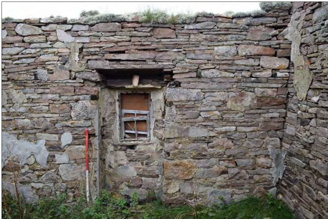
Plate 23: East end of north elevation, Building 1 (North Range) showing former exterior doorway blocked up to form a small window.
