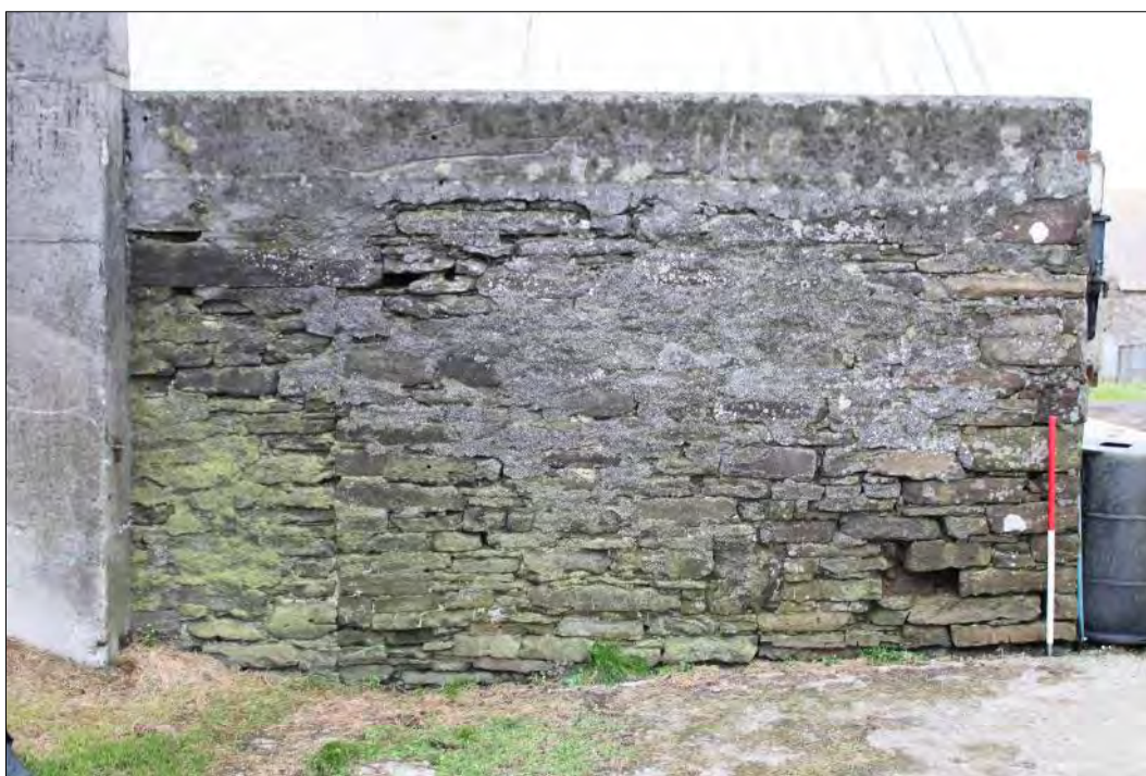
Plate 110: Length of upstanding wall (Building 17) incorporated into a modern agricultural shed, looking southwest. It is possible that this was originally part of a byre shown on the 1844 plan. A blocked doorway or window is visible at the south (left) end.
