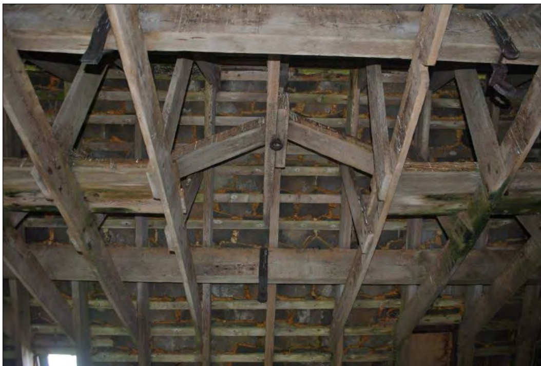
Plate 136: Detail of the roof showing the modified central truss with iron ring (centre) and three iron bands on the timbers around including one with a hook (top right).
