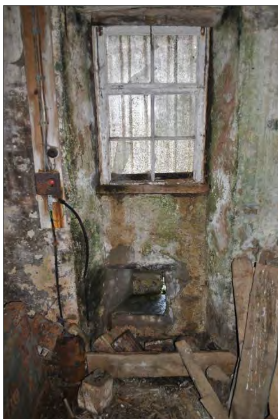
Plate 90: Detail of the west gable of the threshing mill showing the opening cut into the wall below the window.
