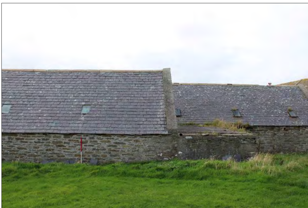
Plate 95: The northeast corner of the turnip shed (Building 9) showing the annex structure butting against the north elevation.
