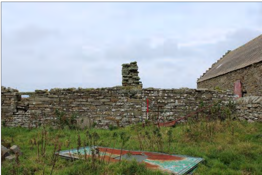
Plate 101: The east end of the south-facing elevation, Building 11, showing the upstanding east gable and the construction break with the annex (Building 11.1).
