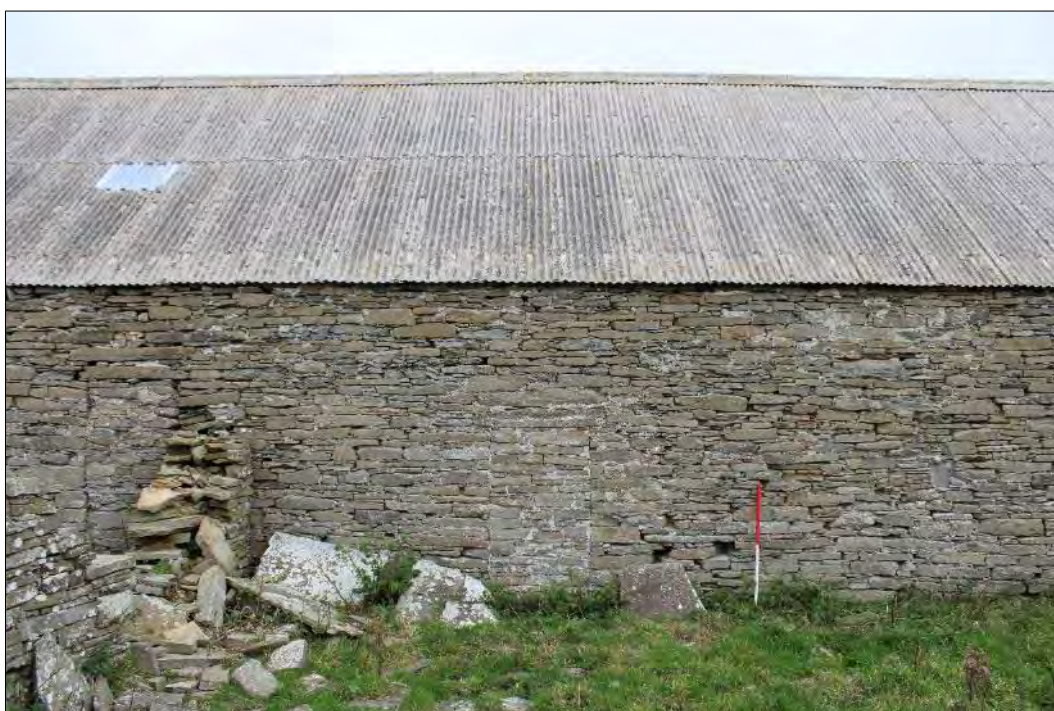
Plate 98: Detail of the west-facing elevation of the old threshing barn showing two blocked doorways. The wall butting against the elevation next to the left doorway is the south elevation of Building 12.1.
