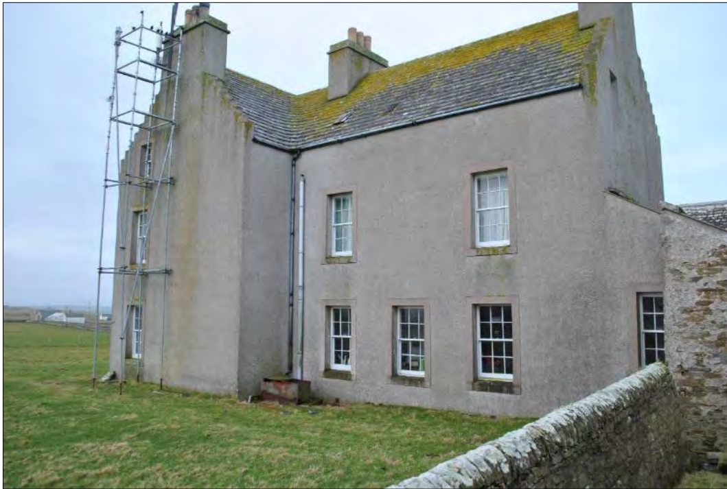
Plate 71: General view of the east-facing elevation of Holland House (Building 3.1) showing a number of architectural features common throughout the building. The lean-to can be seen on the right, butting against the north elevation of the house and shows the contrasting finishes of the domestic and agricultural structures.
