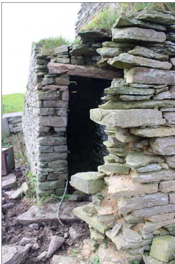
Plate 162: Detail of the staircase butting against the east gable showing the space below the stairs which is accessible from the passage leading to the external doorway.
