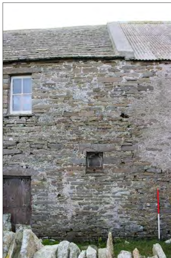
Plate 87: Detail of the north facing elevation, Building 6.2, showing the small window and the external doorway (left) with the grain loft window above.
