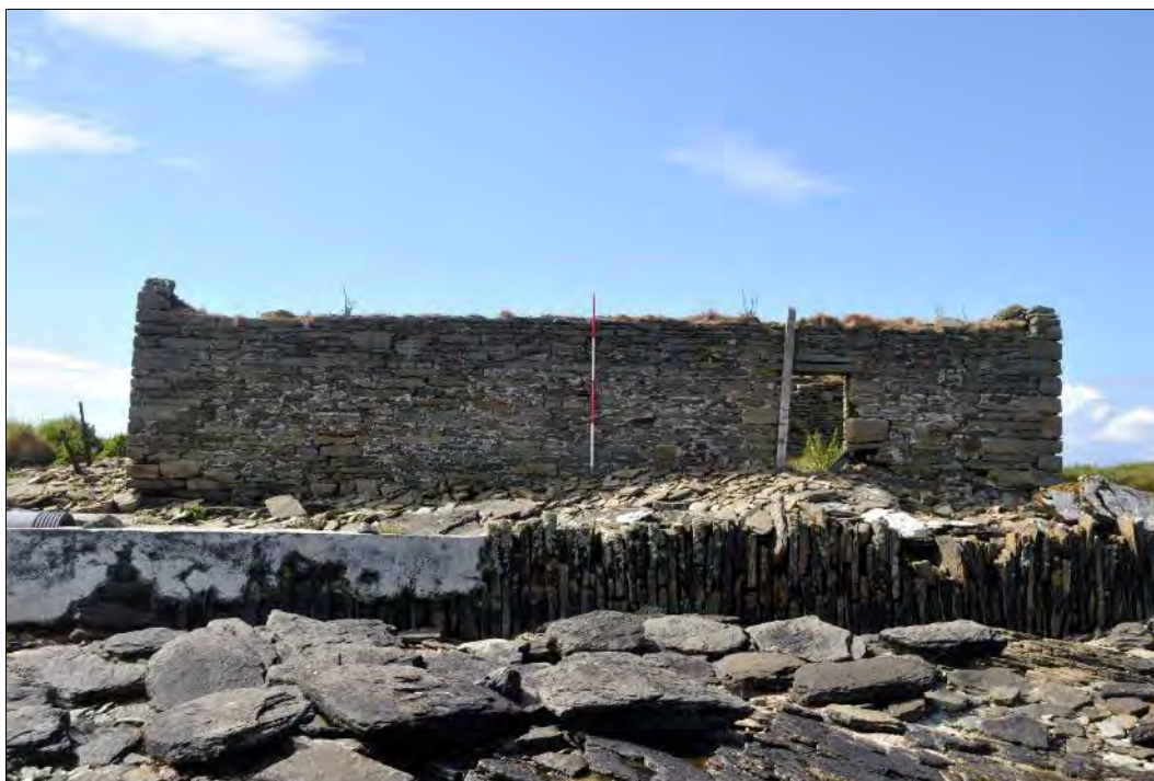
Plate 59: North-facing elevation of Hookin Mill (June 2016) with the vertical flagstones forming the sea wall in the foreground.
