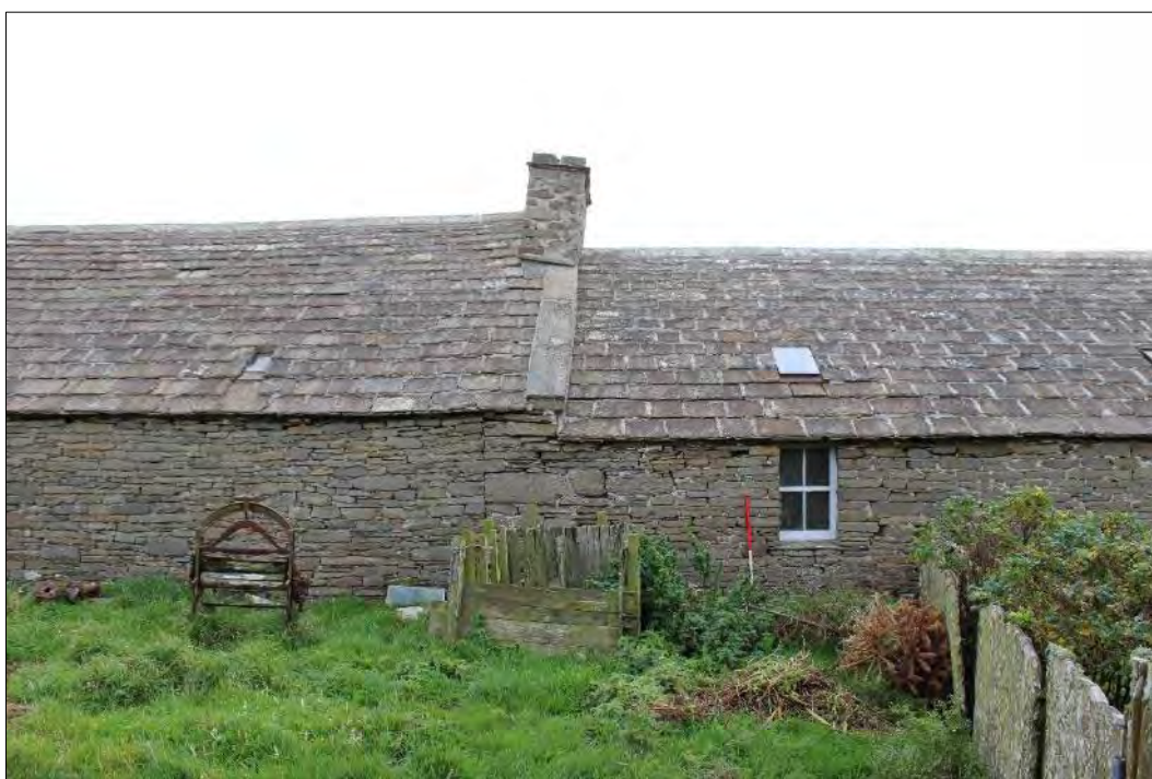
Plate 78: The west-facing elevation of Building 4 showing the construction break between Building 4.1 (right) and Building 4.2 (left). The view also shows how the wall of Building 4.1 aligns with the chimney and the overlapping roof of Building 4.2.
