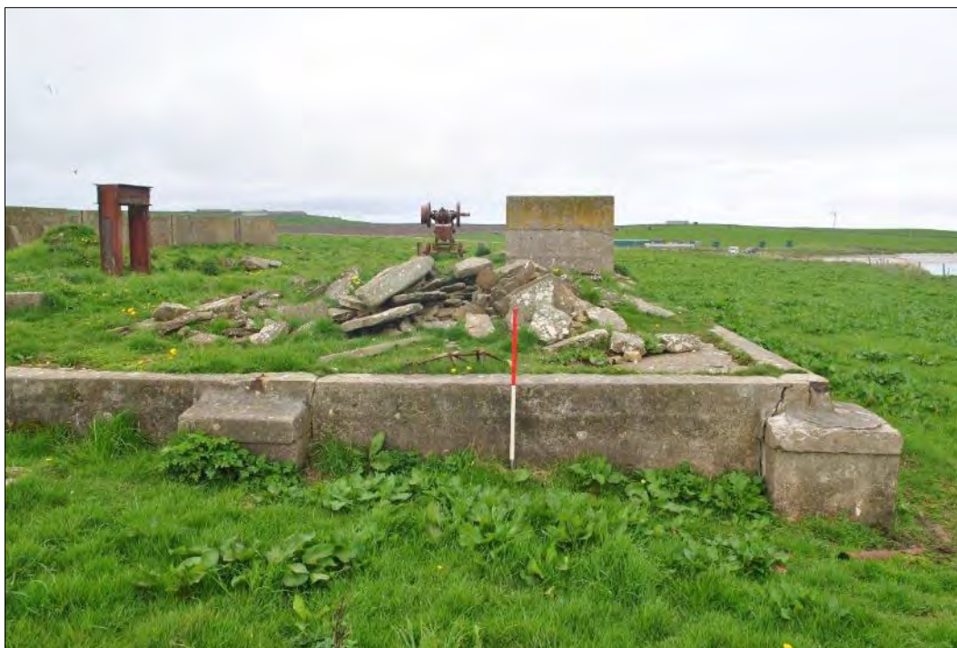
Plate 202: The northeast corner of the concrete platform, looking northwest, with the tank in the background and the iron girder-arch to the southwest (left). The photograph also shows two of the low buttresses which are interspaced around the open sides of the platform. These two examples can also be identified on a photograph of the plant dating from the late 1930s.
