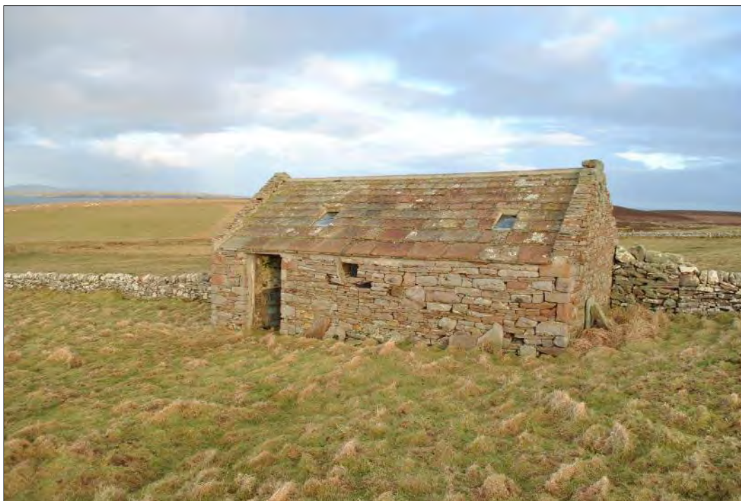
Plate 39: General view of Building 17, looking northwest, showing external doorway and modified opening in the south-facing elevation.
