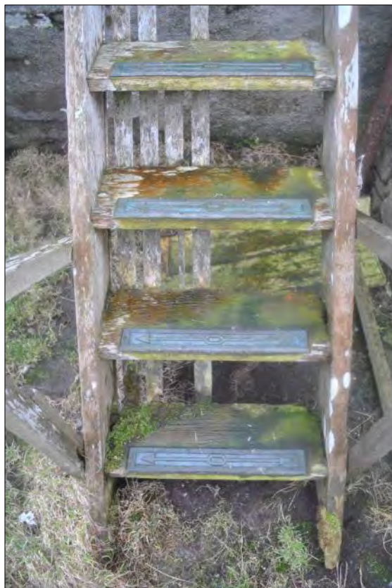
Plate 85: A detail view of the timber staircase which provides access to the platform at the east end of Building 6.
