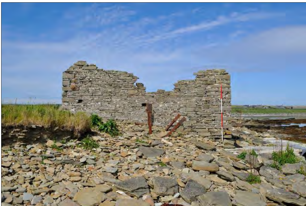
Plate 58: East-facing gable of Hookin Mill (June 2016) with the spokes of the mill-wheel protruding from the pebbled stones filling the wheel pit.
