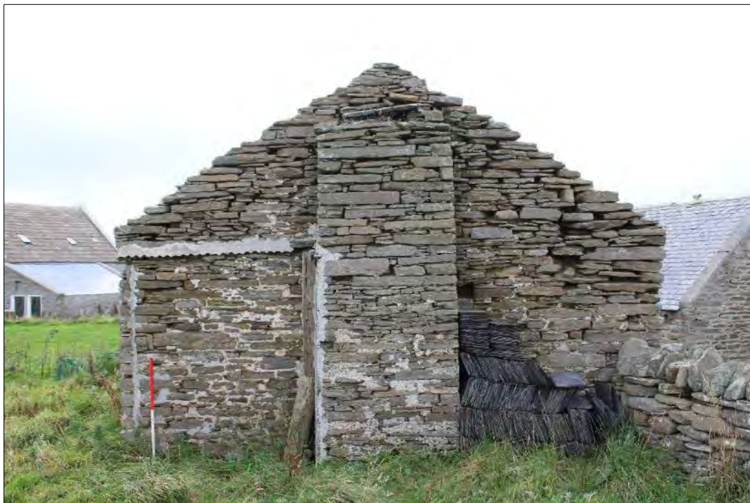
Plate 82: North-facing elevation of Building 5 showing the outstanding chimney lumb and the mortar deposits indicating the former presence of a lean-to with a roof of corrugated material.
