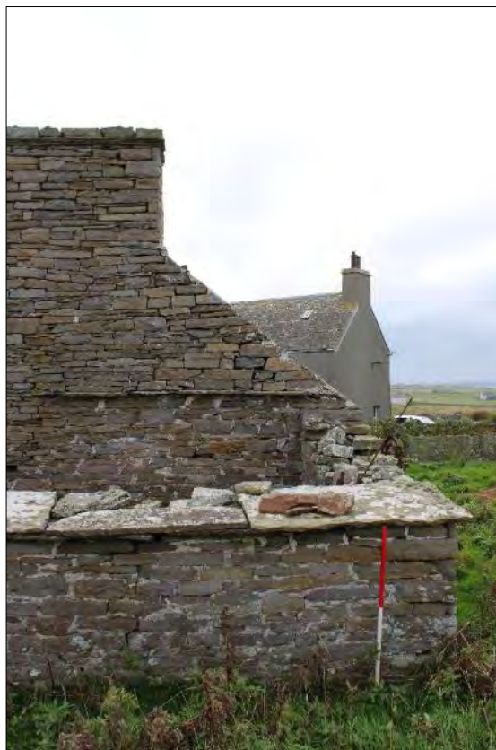
Plate 79: The northwest corner of Building 4.3 looking south, showing the remnants of the flagged roof and the north elevation of Building 4.2 with the line of mortar indicating the former roof line of Building 4.3.
