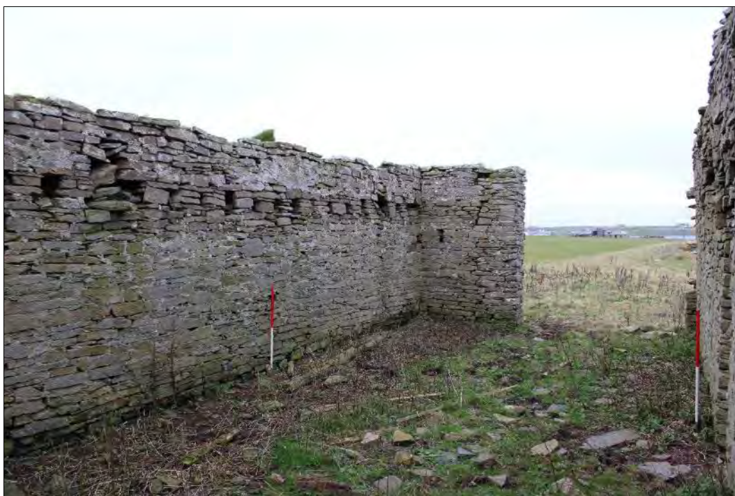
Plate 168: Interior looking north showing the slots for the first floor joists slightly below the truncated wall head.
