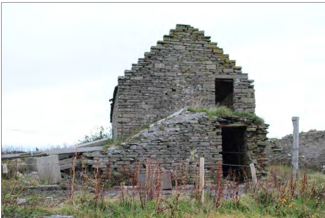
Plate 161: East-facing gable showing external stairs and doorway at ground- and first-floor levels.
