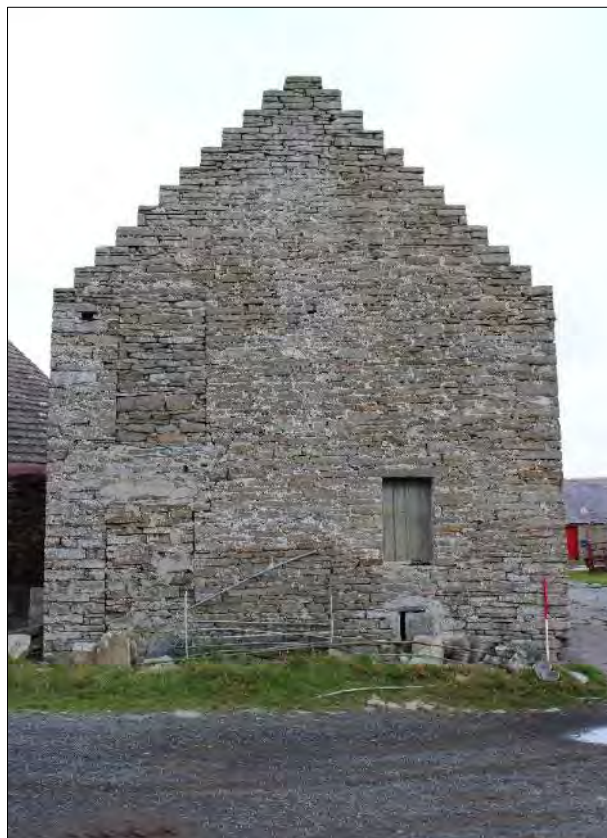
Plate 89: West gable of the threshing mill (Building 6.3) showing the blocked doorways (left) and window (right) with an opening below.
