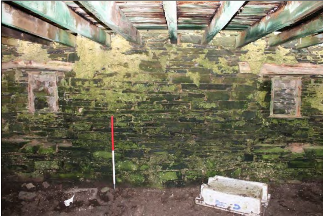
Plate 163: South elevation with blocked windows.
