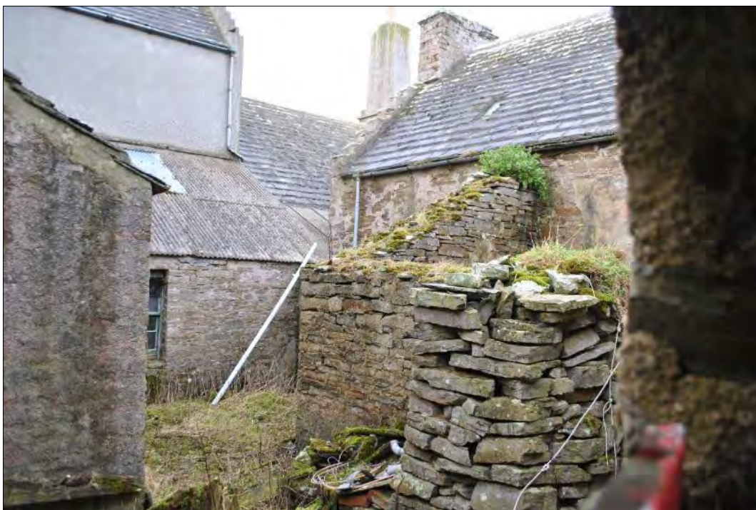
Plate 72: The courtyard at Holland House looking southwest through the partially blocked courtyard entrance. The north-facing elevations of the south wing and the service wing with a lean-to structure obscuring the ground floor level are in the right and centre background. On the right is the earlier structure, Building 3.2, with the roofless remains of another lean-to structure butting against its east-facing elevation.
