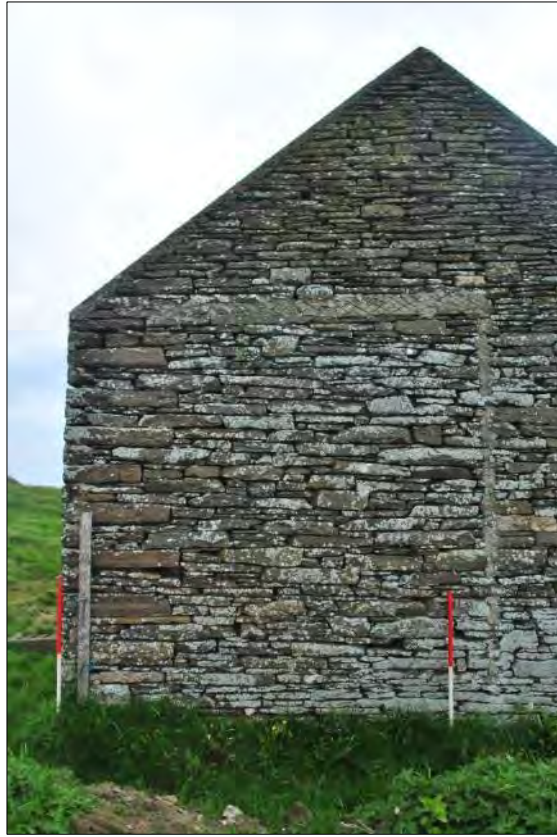
Plate 131: North side of the west-facing gable showing the L-shaped deposit of mortar.
