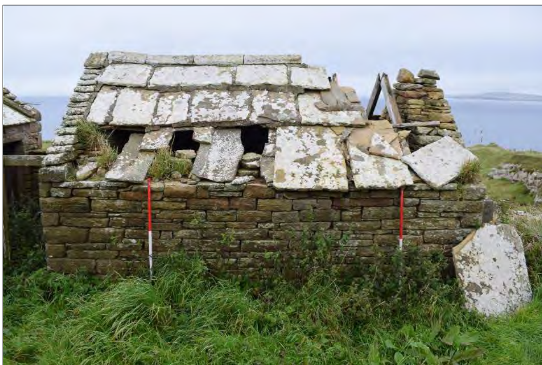
Plate 178: South-facing elevation of Building 6 showing partially collapsed roof.
