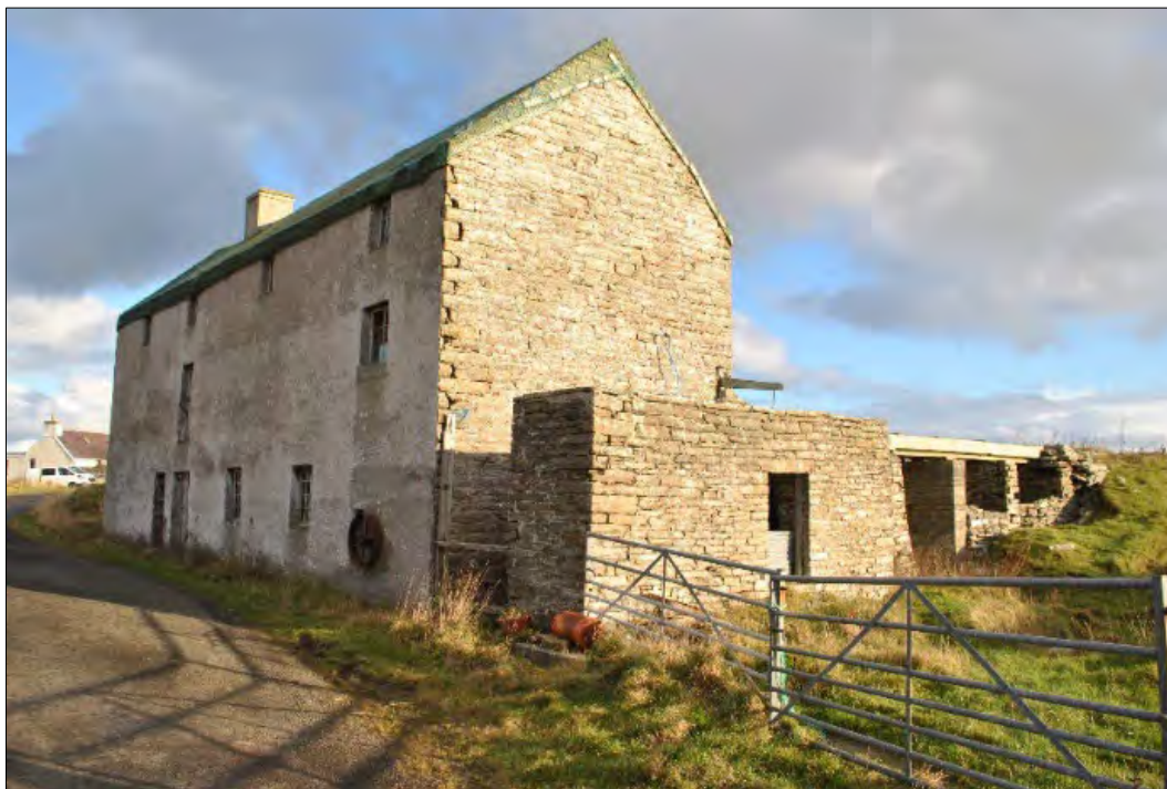
Plate 144: View of Meikle Meal Mill, Stronsay, looking east, showing the harled front (northwest-facing) elevation and the roofless structure against the southwest gable housing the water wheel.
