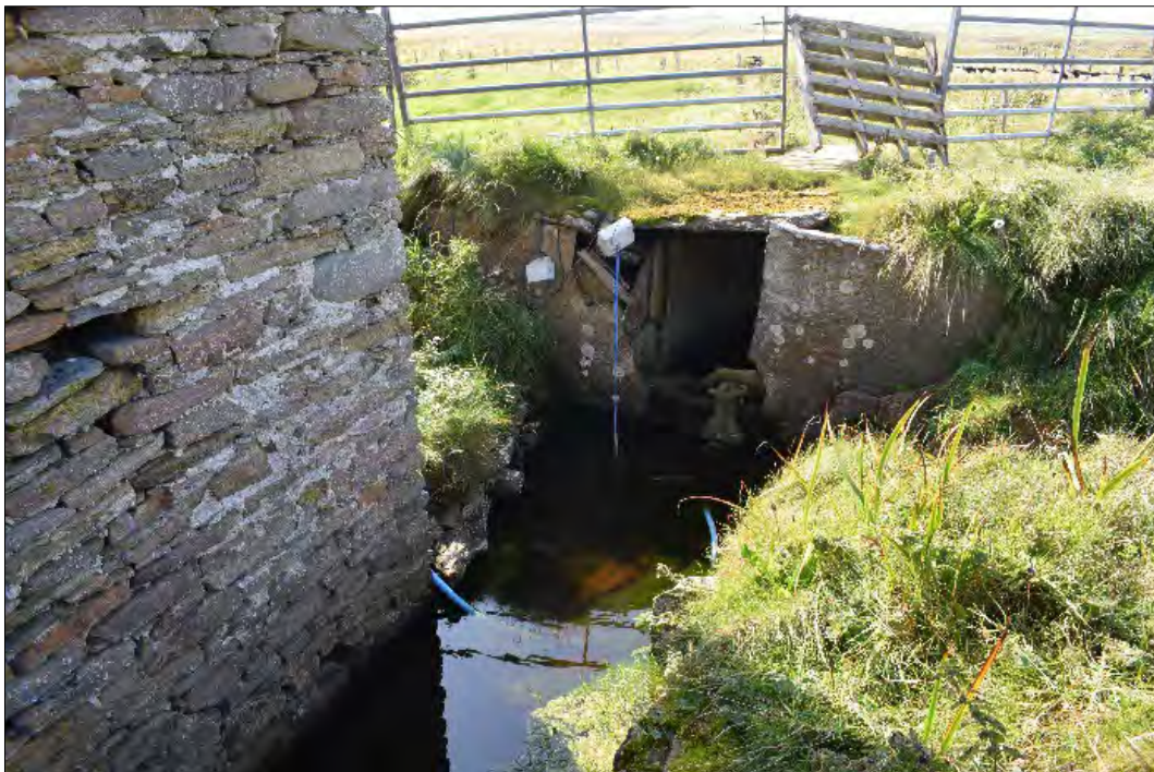
Plate 46: General view, looking southwest, showing the stone-lined mill race at the south end of the wheel pit.
