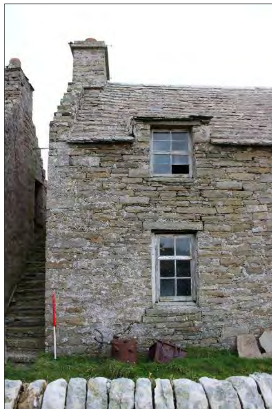
Plate 66: The west end of the south-facing elevation, Building 1 showing the ground floor window and the first floor wall dormer. The stairs butting the west gable (left) provide access to the first floor of Building 2.
