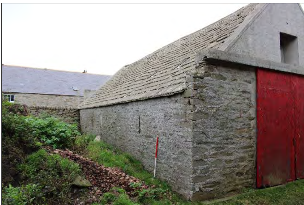
Plate 109: General view of Building 15, looking southeast, showing the differing ground surface levels at the west (foreground) and east ends (background).
