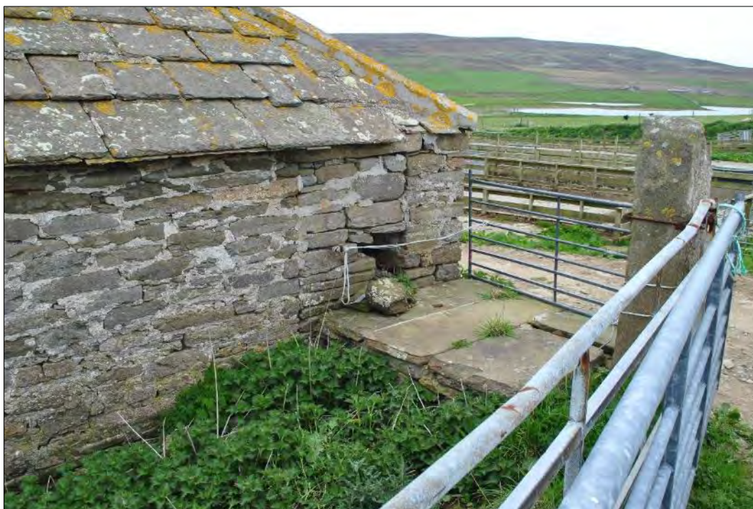
Plate 128: West end, north-facing elevation of FB 12 with the stone-built platform butting against the lower edge of a blocked window.
