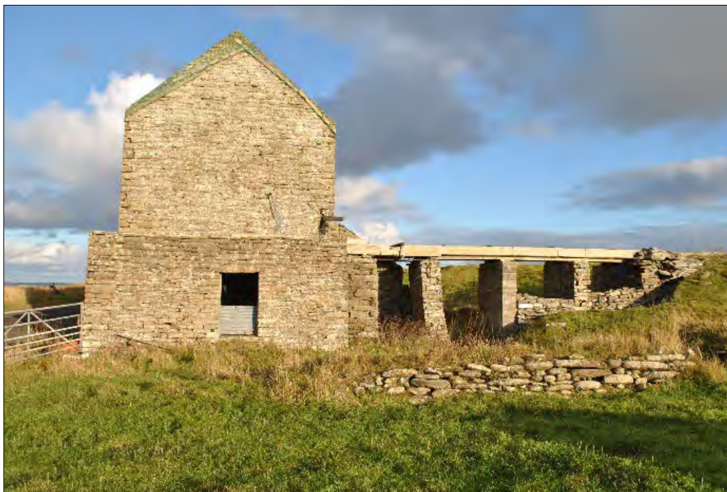
Plate 156: Southwest gable of the mill showing the timber trough supported by four pillars and the roofless water wheel house. The timber beam operating the sluice above the water wheel is visible protruding from the gable. The dry-stone walling in the foreground marks the approximate south edge of the overflow ditch.
