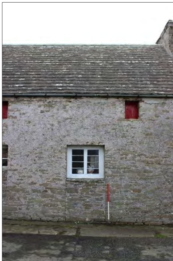
Plate 74: Detail of the west-facing elevation, Building 3.2 showing the former external doorway partially blocked to form a ground-floor window.
