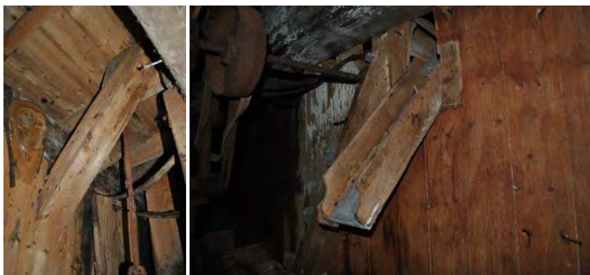
Plate 146: Two views of a chute descending from the first floor of the mill and passing through the partition at the southwest end of the main ground floor room. The meal would have passed through a sieve and screen and into a bag.
