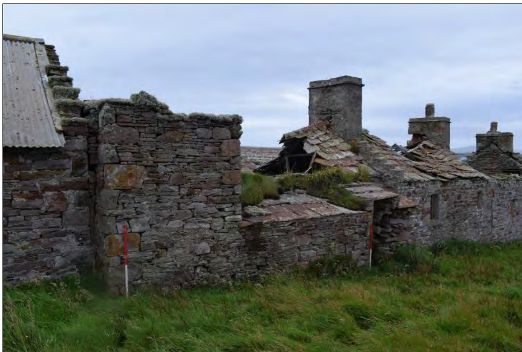
Plate 27: North-facing elevation of north range showing Building 4 comprising a square-plan corn drying-kiln (centre left), looking southwest.
