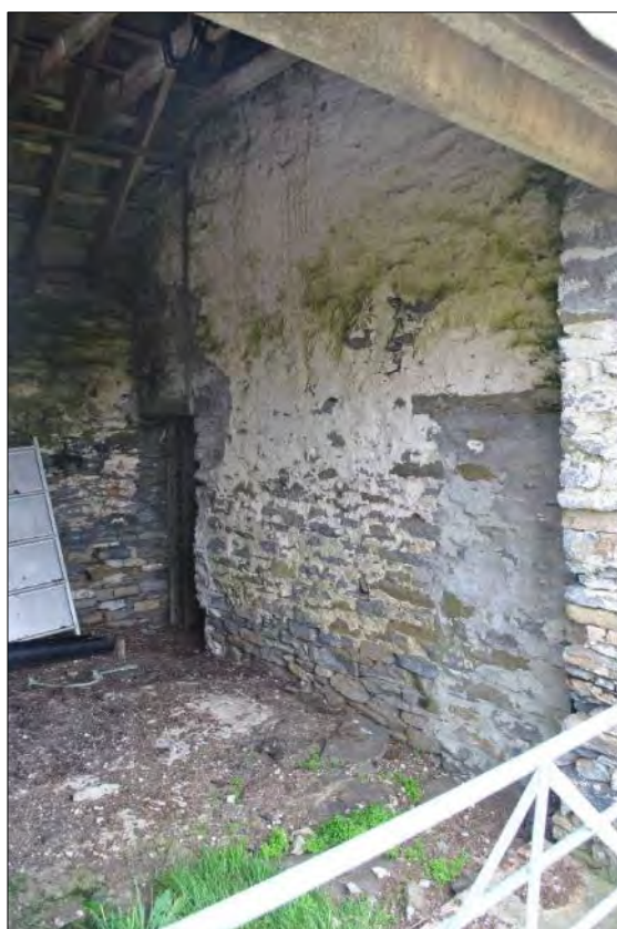
Plate 127: View through doorway in the west-facing elevation of FB 11 with the internal wall marking the point where the building becomes a two storey-structure.
