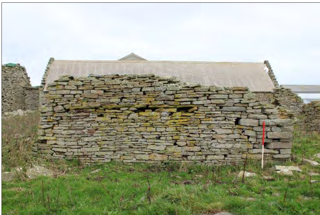
Plate 105: The west-facing (exterior) elevation of the enclosure wall between Building 11 and Building 12 showing the possible re-build at the south end (right). Also visible at the base of the north end are the four course of stonework which appear to butt against the southwest corner of Building 12.
