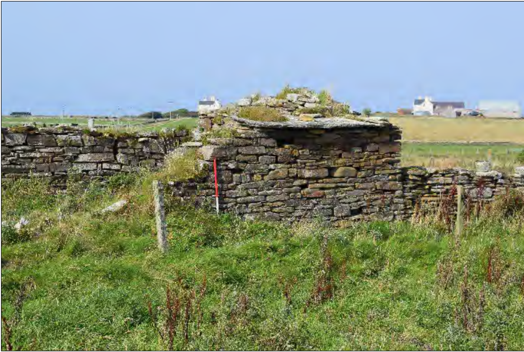
Plate 51: Northeast corner of building to east of the later mill, looking northwest, showing the surviving fragment of a flagstone roof.
