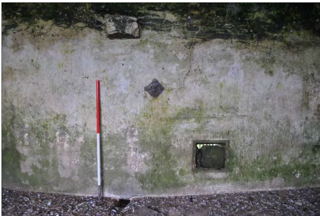
Plate 135: South elevation with surface drain at the foot of the wall and chamfered protruding stone directly above.
