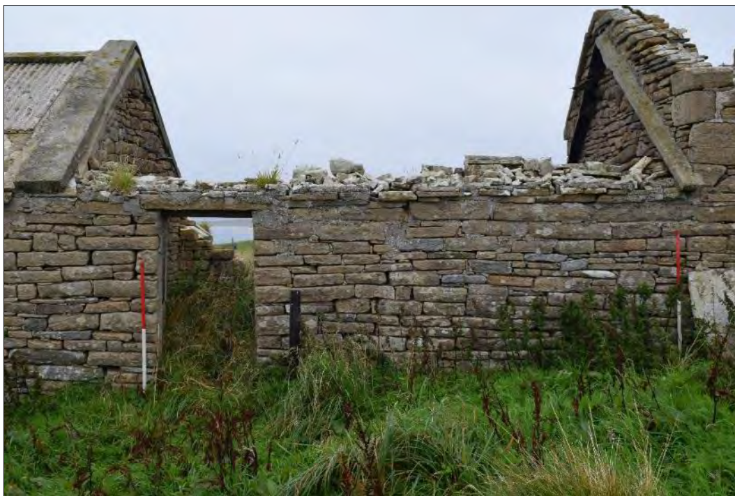
Plate 176: West-facing elevation of Building 3 showing the line of the roof on the shared gable with Building 2 (right) and the external doorway.
