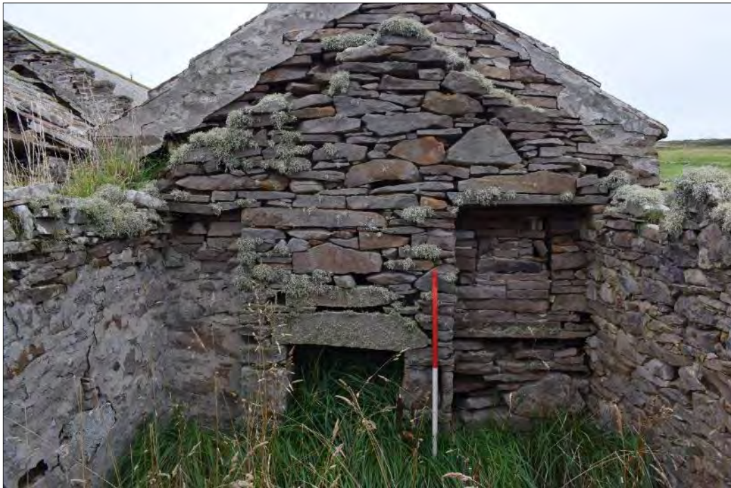
Plate 32: East elevation of Room 8 with the west-facing gable of Building 7 behind showing possible blocked doorway to the right (south) of the fireplace.
