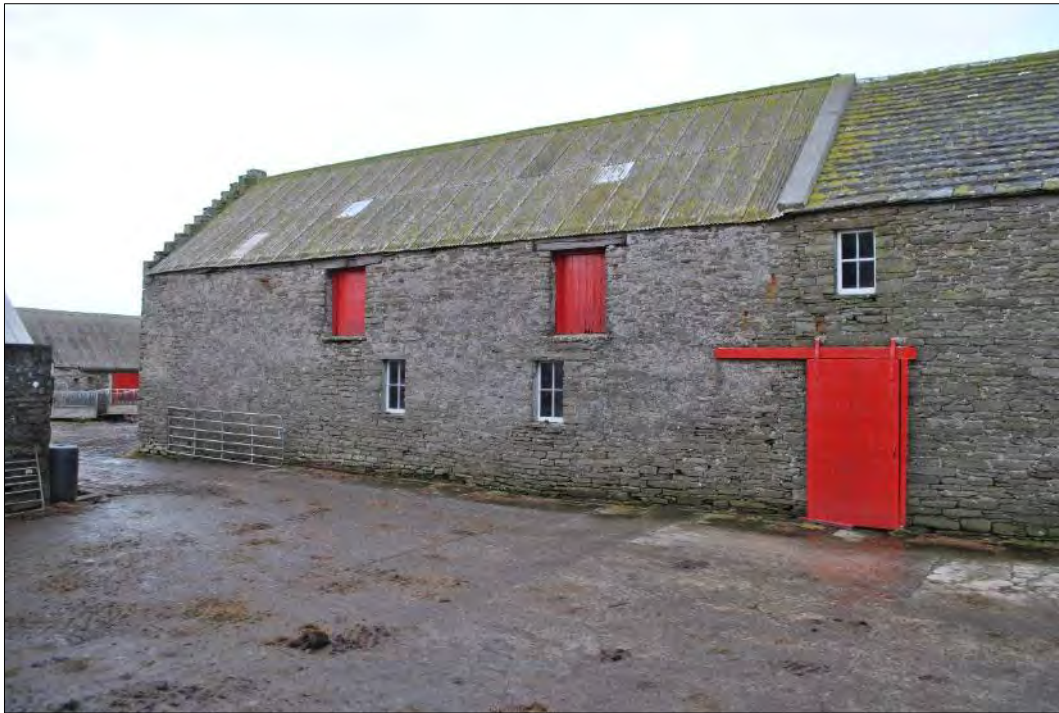
Plate 88: General view of the south-facing elevation of the threshing mill (Building 6.3) showing the first floor external doorways. The sliding door on the right provides access to Building 6.2.
