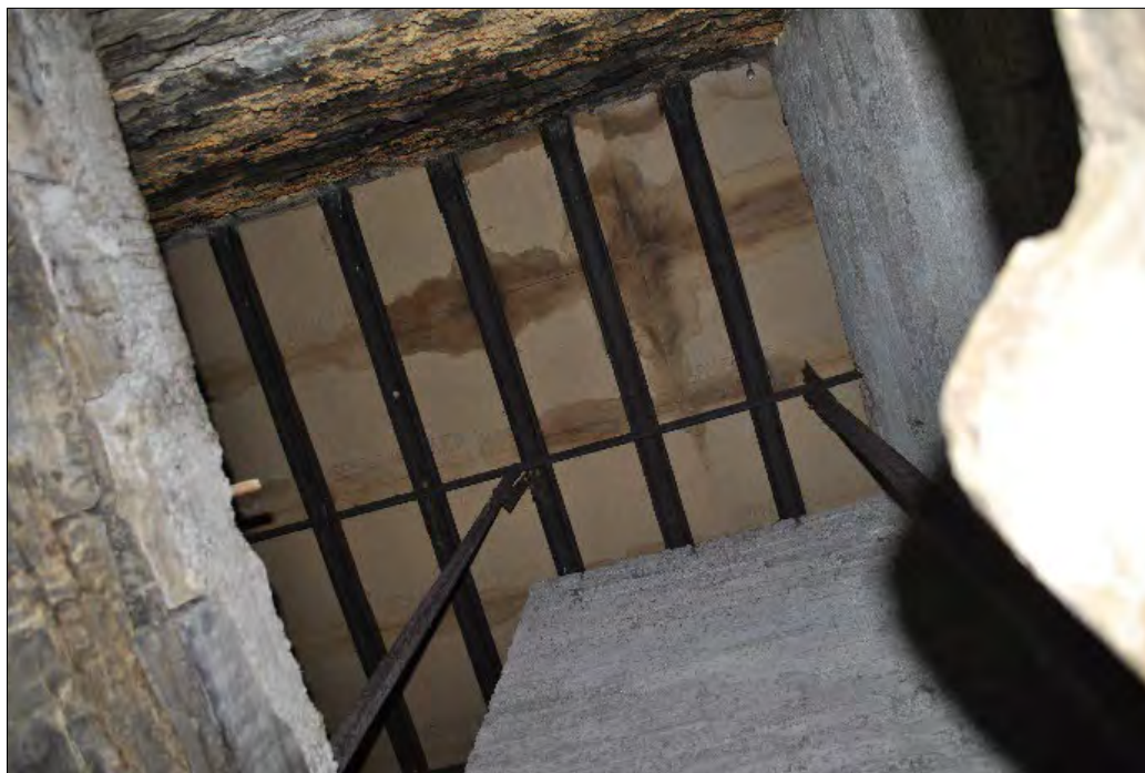
Plate 151: View looking up from the ground floor of the corn-drying kiln at the underside of the replacement flooring of the second floor. The cross-beams appear to be iron and are probably the original fittings that formed part of the drying floor. Also visible are modern alterations to the upper structure of the kiln itself.
