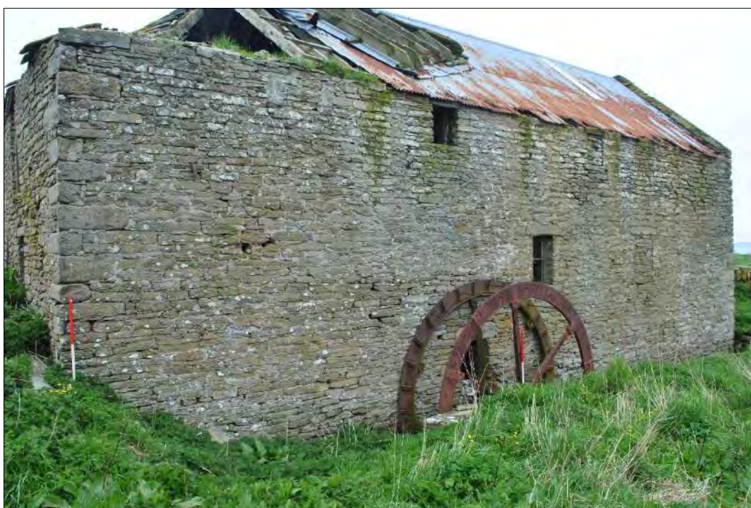
Plate 125: South-facing elevation of FB 10.3 showing the three internal levels and the mill wheel.
