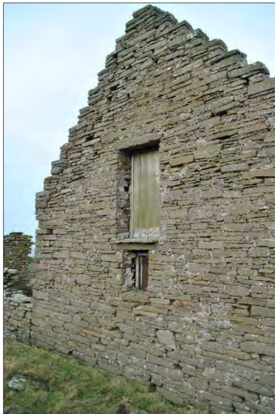
Plate 97: South gable of the old threshing barn (Building 10) with doorway at loft height and window below. The blocking between Building 10 and Building 11.1 can be seen on the extreme left of the photograph.
