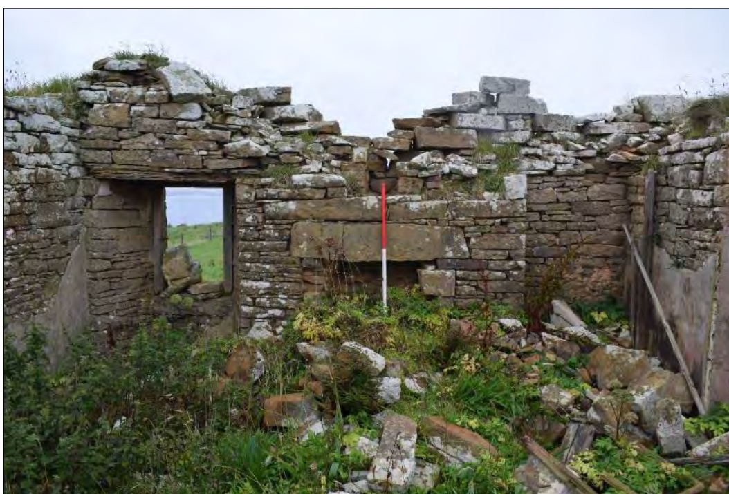
Plate 174: East elevation, Building 1 at Quarryhouse with centrally-placed fireplace, storage cupboard (right) and external window.
