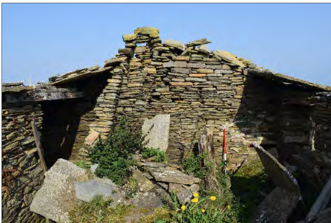
Plate 53: Interior north gable of former smithy showing scar of forge chimney breast in the stonework.
