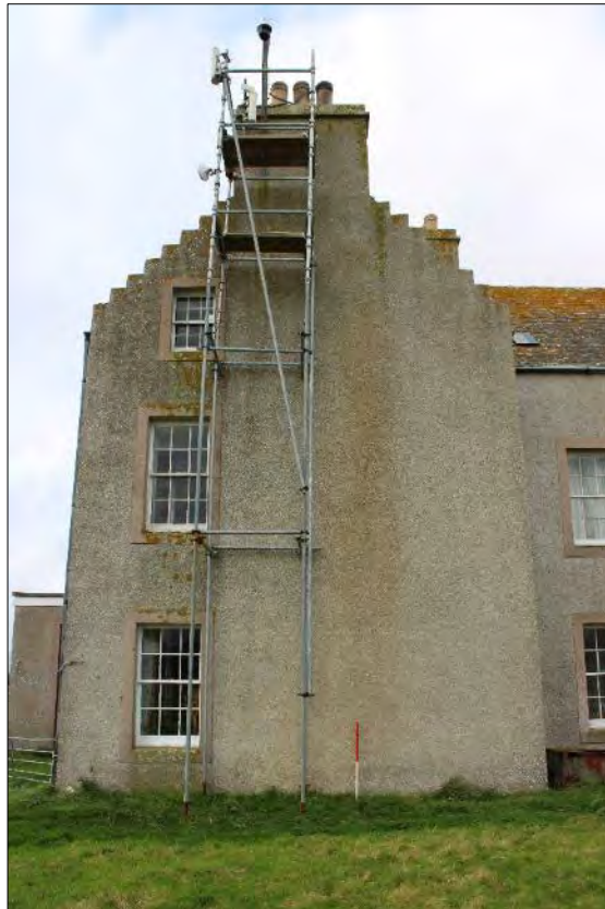
Plate 70: The east-facing gable of the south wing, Holland House showing the ground and first floor windows, and the smaller attic window. These are all positioned towards the left of the space that, internally, would contain the fireplaces and flues associated with the chimney at the top of the gable end.
