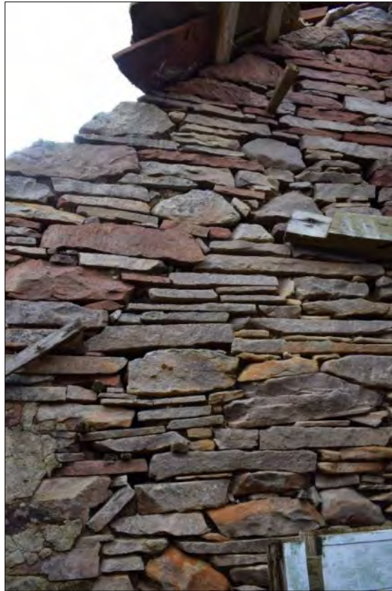
Plate 22: Detail of dividing wall (east elevation) viewed from Building 2 showing construction scar which appears to demarcate the original line of the gable roof line with the lumb rising from it.
