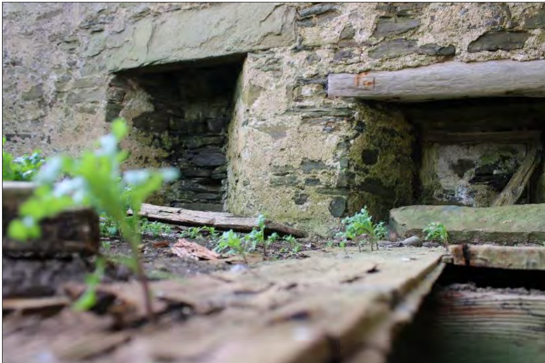
Plate 164: Detail of west elevation, first floor with fireplace (left) and blocked window (right).
