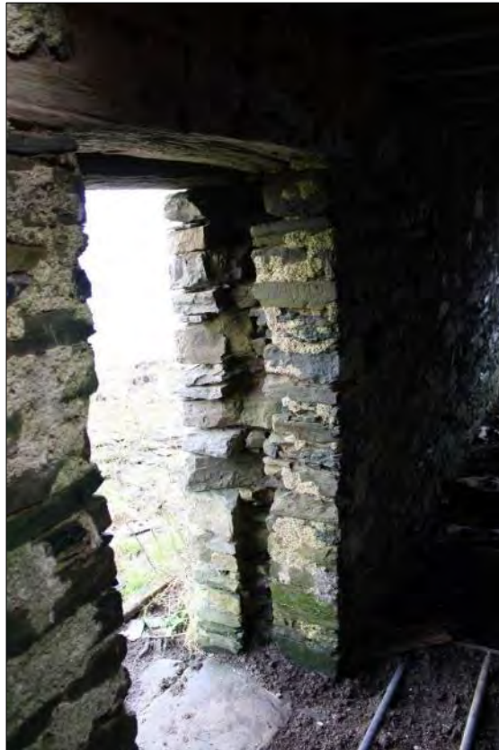
Plate 160: Detail of external doorway in north-facing elevation with a wall scar showing the former position of the door frame.
