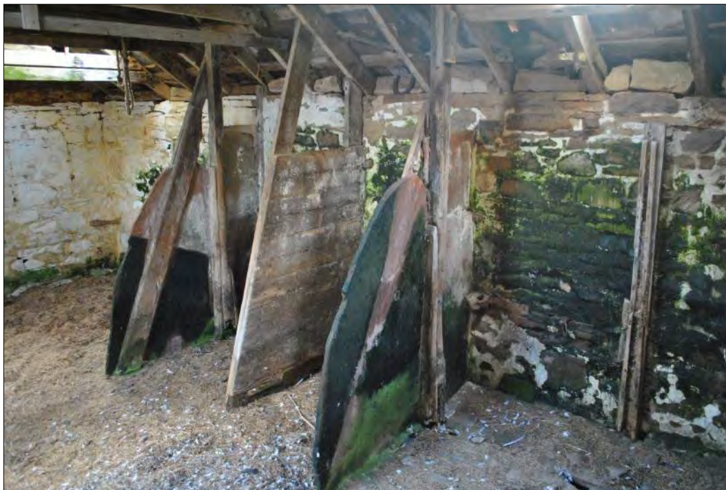
Plate 36: Interior of Building 17 showing the extant byre fixtures. The second divider is timber-built with the two flanking dividers being predominately red sandstone slabs held in position by timber supports.
