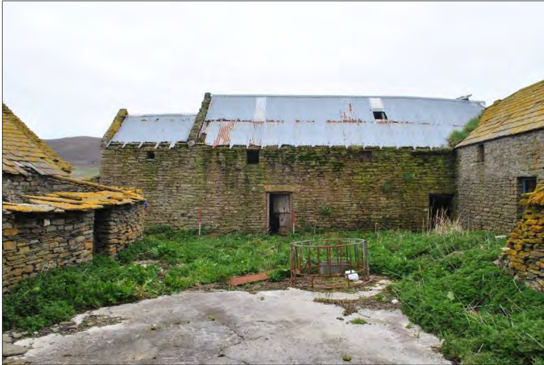
Plate 123: North-facing elevation of FB 10, with FB 9 (left) and FB 11 (right), showing the two exterior doorways and first-floor windows in FB 10.3 (centre and right), and the widow in FB 10.2 (left end). The lean-to structure FB 10.1 is obscured by FB 10.1.
