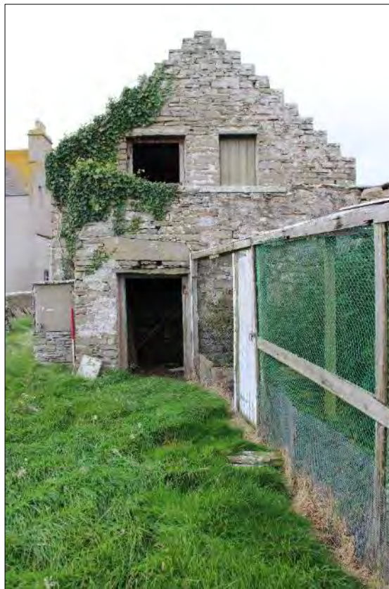
Plate 67: East-facing gable of Building 1 showing first floor external doorway and window with, below, a doorway providing access to the storage space under the stone stairs.
