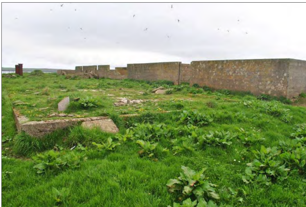
Plate 201: A closer view of the plant showing the walling and the opening providing access to the internal areas. The northwest edge of raised concrete platform is visible in the foreground.
