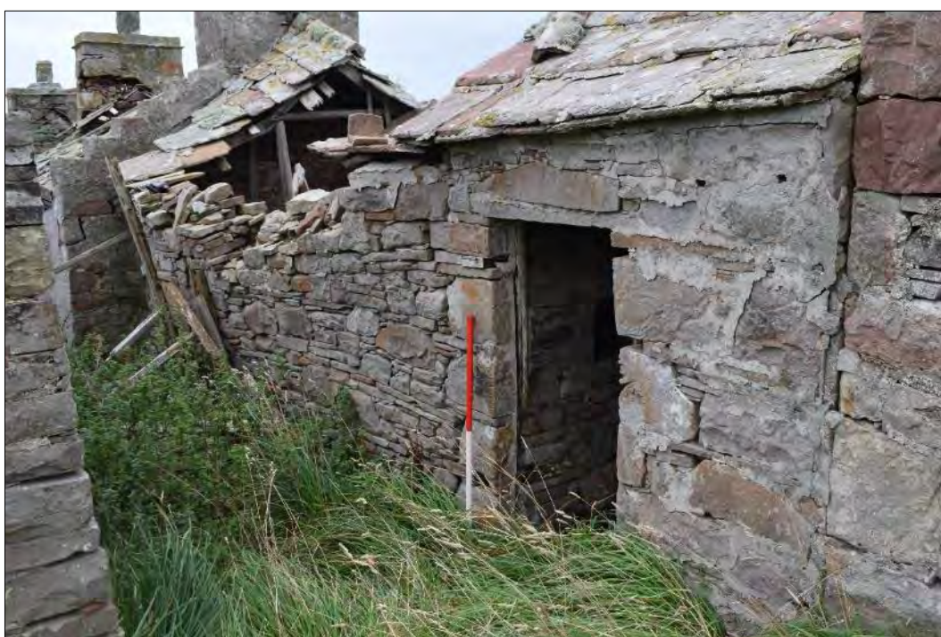
Plate 25: South-facing elevation of Building 3 (left of centre) with collapsed roof and bowing wall butting against the gable end of Building 2, and Building 4 (right), looking northwest.
