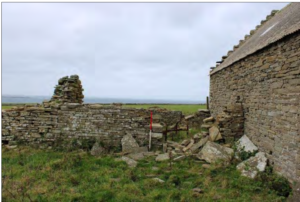
Plate 103: The annex to Building 12, looking north. The doorway is visible to the right of the upright scale and the left side window in the wall beyond is also discernible. The walls of the annex can clearly be seen to butt against both Building 10 (right) and Building 12.
