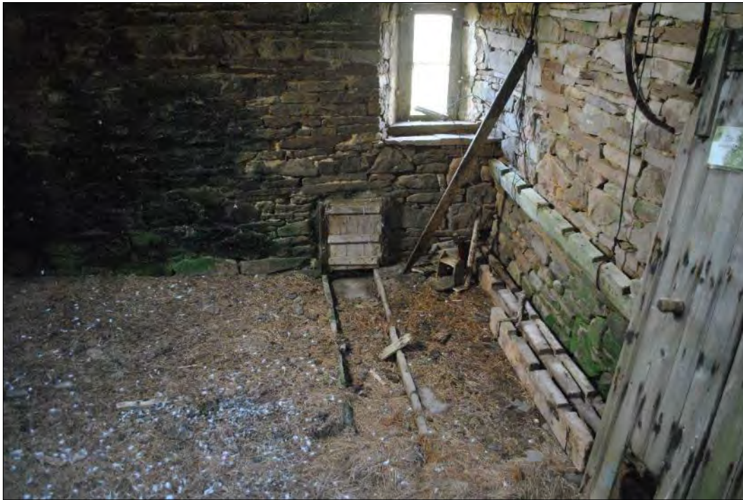
Plate 37: The northwest corner of Building 11 with the floor surface drain flowing into the oodle hole at the base of the west elevation.
