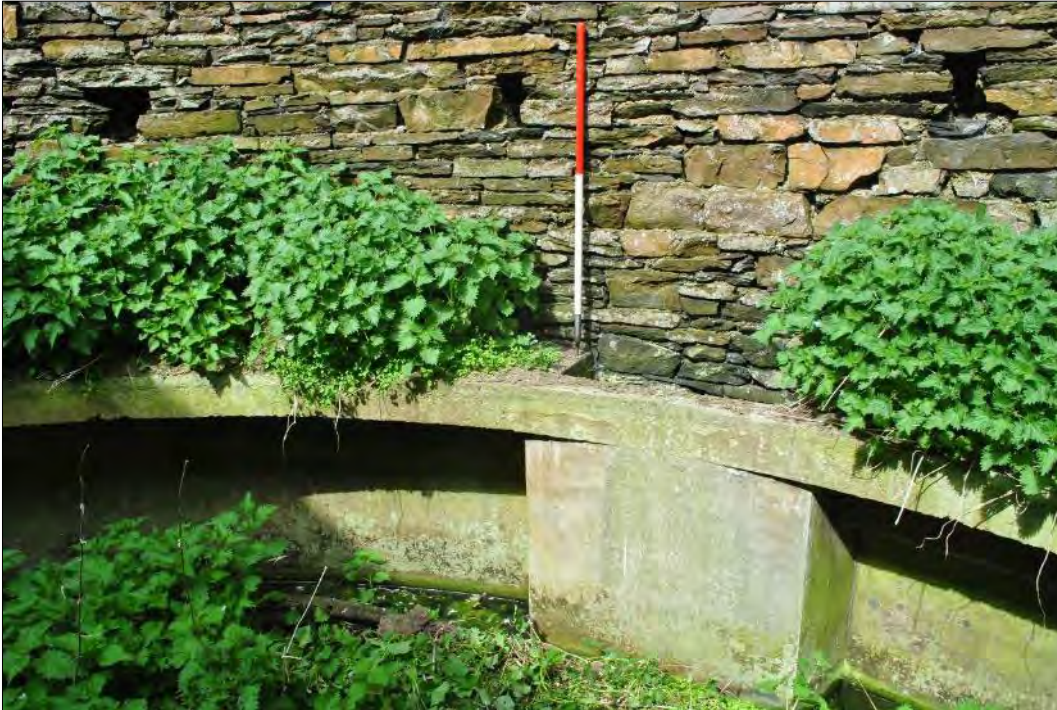
Plate 142: The concrete ring running around the base of the of the interior wall. The metal ring which runs inside of this is visible in the nettles at the bottom of the picture.
